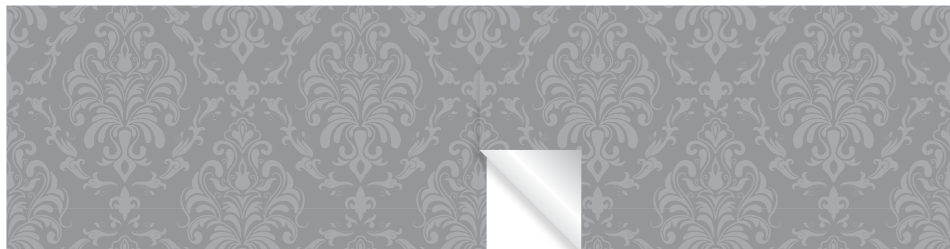
Wallpaper installation misalignment with overlap
